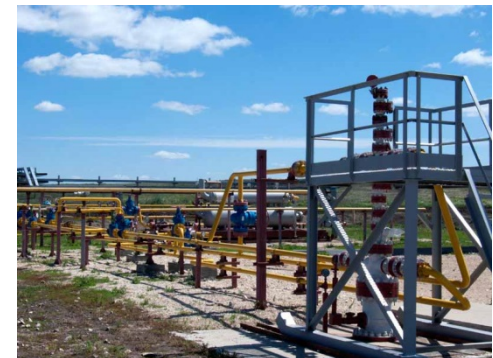
VM#1 wellhead and flow line
