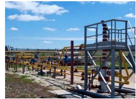
VM#1 wellhead and flow line
